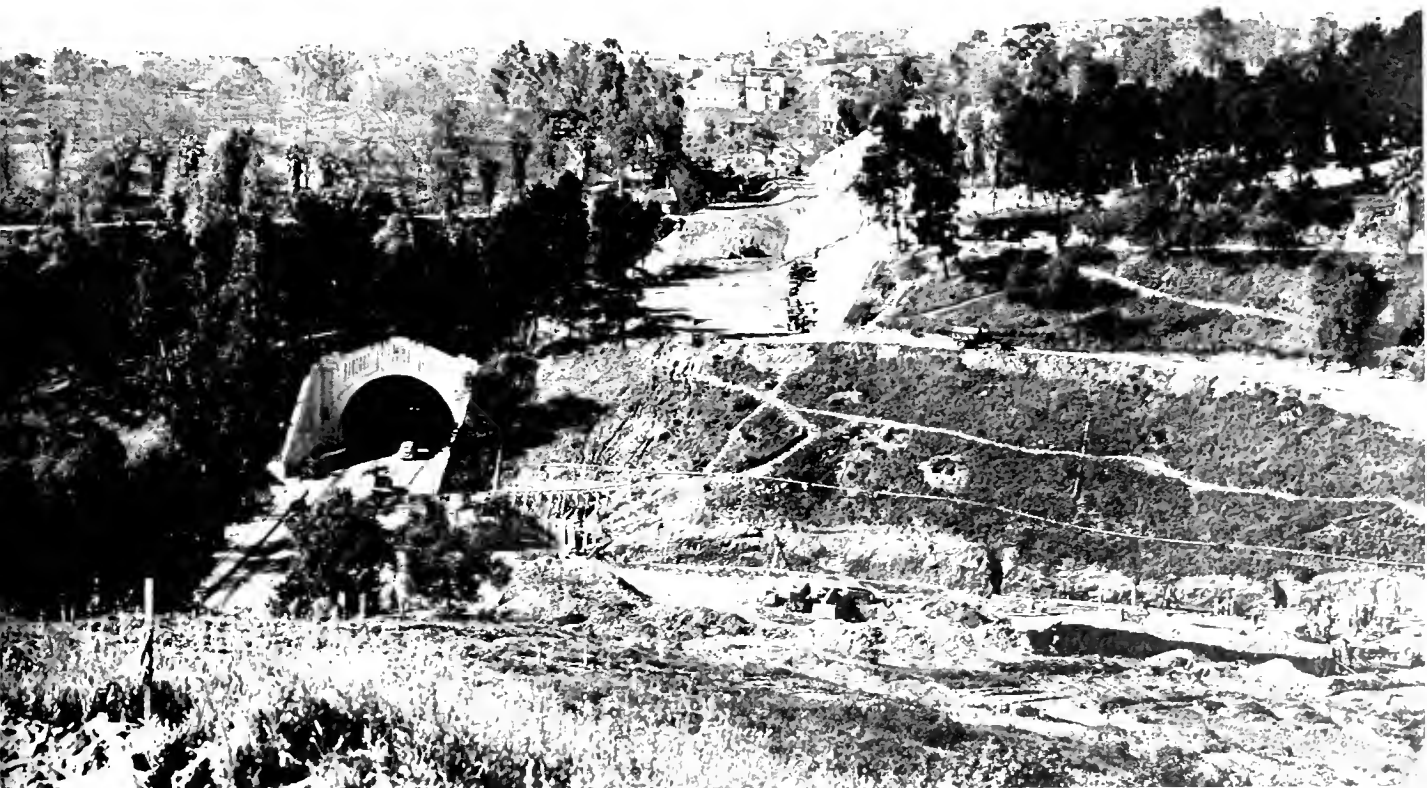
Open cut construction parallels existing Figueroa Street tunnels for northbound traffic seen at left. Large fill will be built in foreground
